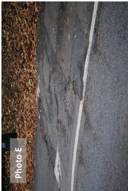
Point 7 on map The speed bumps are poorly maintained and ineffective to large vehicles, particularly the large plant vehicles travelling through the village.
